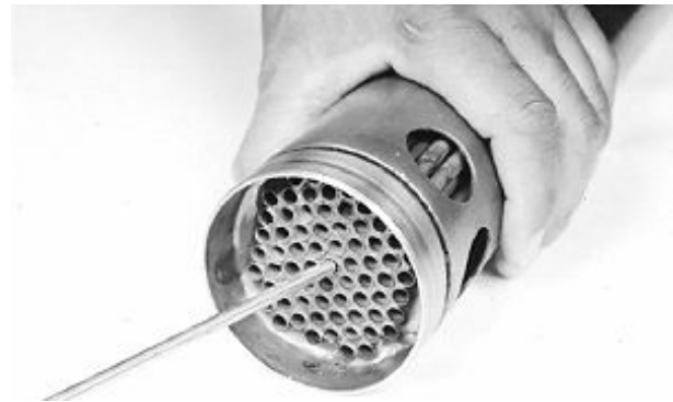
Clean Heat Exchanger
